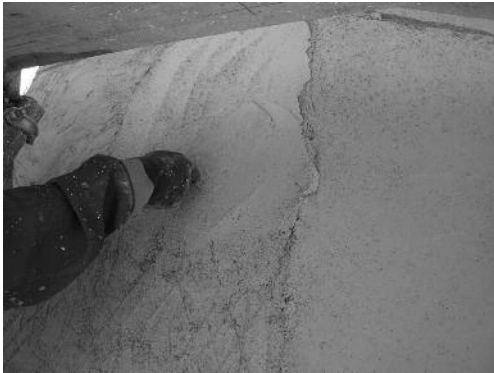
Fig. 11 Application of the restoration lime mortars, after the humidification of the support. Scattering until the render thickness was obtained.
