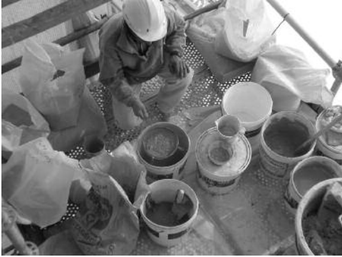
Fig. 10 Preparation the restoration lime mortar, mixed with washed sand and standard grain size.
