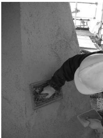
Fig. 12 Using the mason's mortar-board to compress the mortar; before adding different coloured sands to the mortar, and with the mason's mortar-board compressing again the render.
