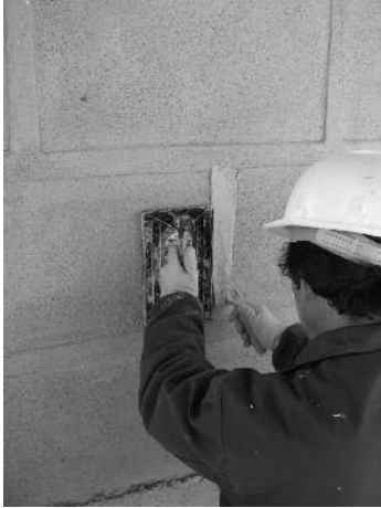
Fig. 22 Applying a thin grain size mortar in the joint area after pressing and watering the render during the drying stage to avoid the mortar being fissured.
