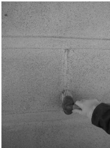
Fig. 17 Removing the mortar in joints with metal tools; cleaning and humidifying the furrows.
