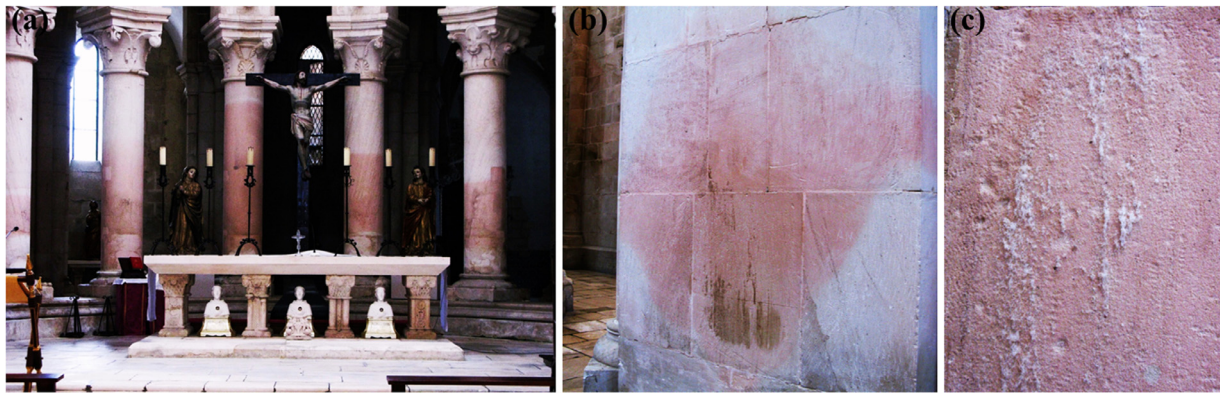
Fig. 1. (a) distinct phenomenon observed at the altar of the monastery church; (b) pink coloured biofilms on the walls; (c) evidence of the presence of salts on the walls.
