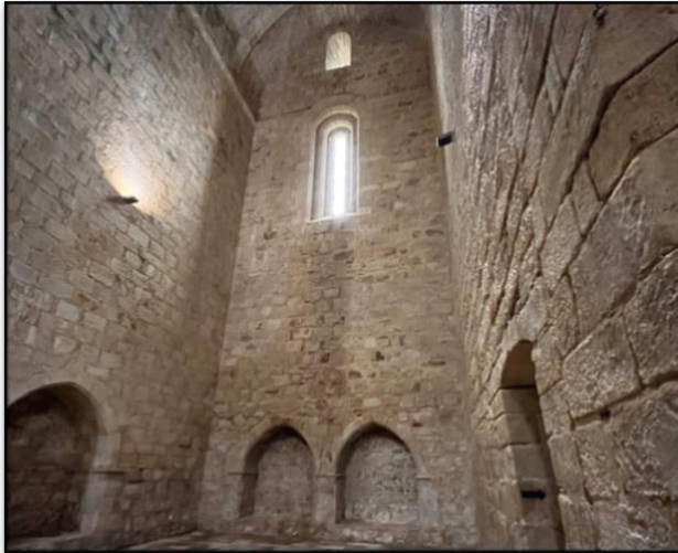
Figure 5 Interior view of the church By LuizaSerpLopes - Own work, CC BY-SA 4.0, https://commons.wikimedia.org/w/index.php?curid=116257883
