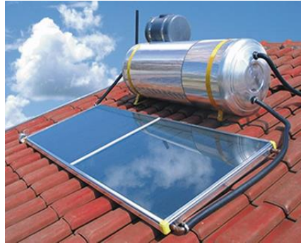
Figure 1.1.3: Solar thermal collectors for water heating installed on the roof. [4]
