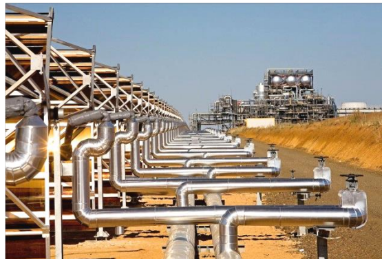
Fig. 1. View of pipes in a 50 MW PT field (Spain).
