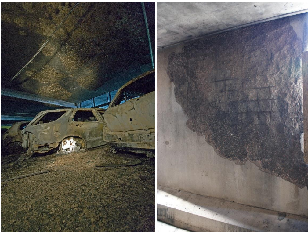
Figure 1 Fire spalling of concrete in parking garages. The heat source in the left picture was five burning cars and in the right picture three burning cars. (Photo Robert McNamee)
