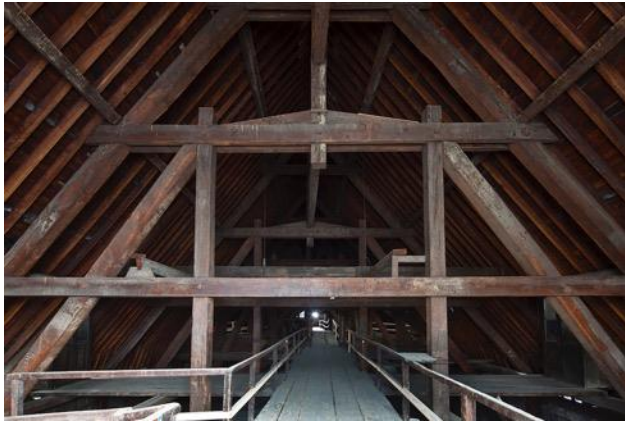
Figure 8 This is the under-drawing of the Notre Dame Roof before the fire. It can be replicated in ferrocement to give the same appearance, density and strength as the original oak roof timbers.
