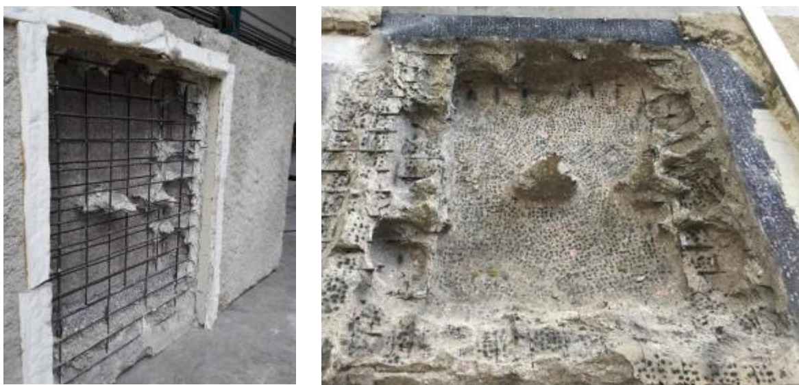
Figure 9 Concrete slab 5 after 52 min exposure in mobile furnace and cooling. Before removing the reinforcing bars (left); after removing the reinforcing bars (right)
