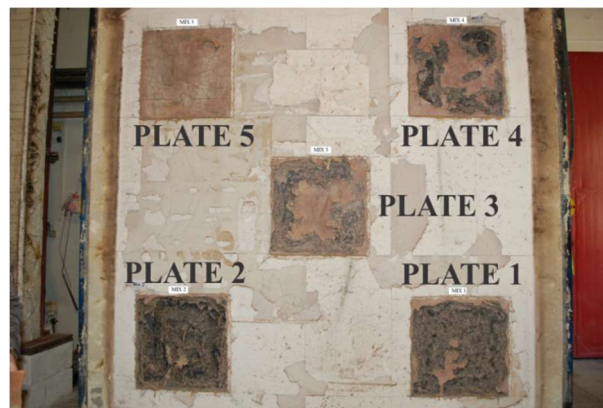
Figure 3: Exposed side of the front cover of the furnace after the fire test with visible spalling damage of the 5 plates.
