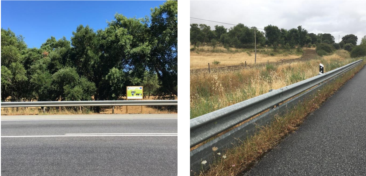
Figure 3: example of a single (left) and double (right) guardrails in the study area
