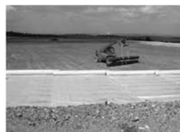
Installation of the Polyfelt® TS20 geotextile separator prior to placement of the granular drainage blanket
