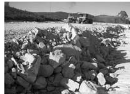
Type of stone fill used as the working platform on top of the Polyfelt® PEC400 geocomposite reinforcement
