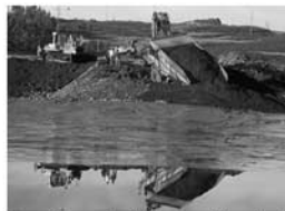
Very soft, saturated tailings at certain locations in the tailings pond
