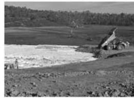
Placement of the granular fill working platform over the Polyfelt® PEC400 geocomposite reinforcement
