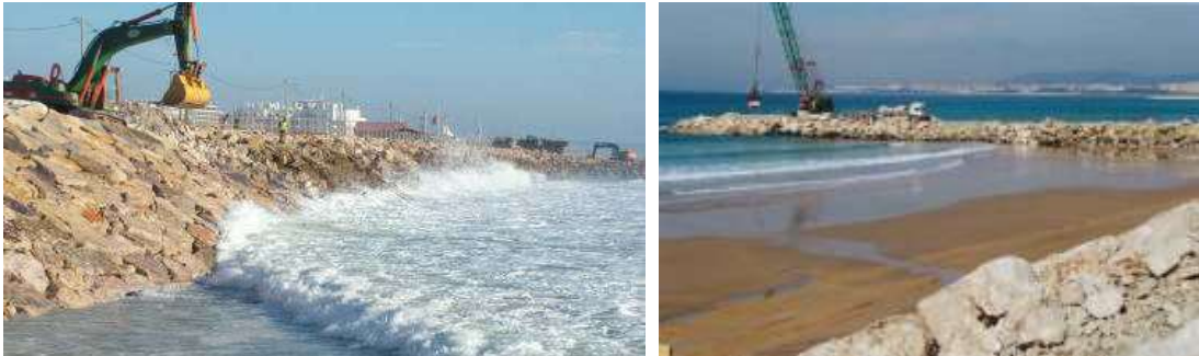
Figure 15: Intervention performed for the repair of spurs and adherent longitudinal work (2004 to 2006)
