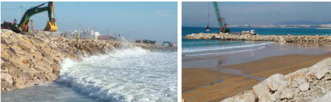
Figure 13: Intervention performed for the repair of spurs and adherent longitudinal work (2004 to 2006)
