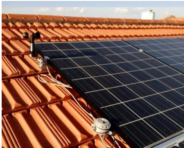
Figure 5. Pyranometer and anemometer installed on the roof.
