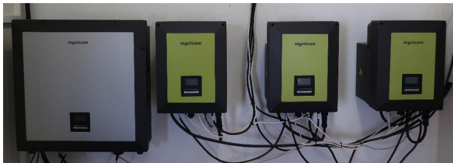
Figure 13: Inverters at the VRFB microgrid: PV inverter (gray), EMS Home bat. inverters (green)
