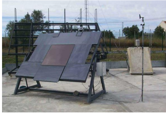
Fig. 16. PV system formed by one amorphous solar module.
