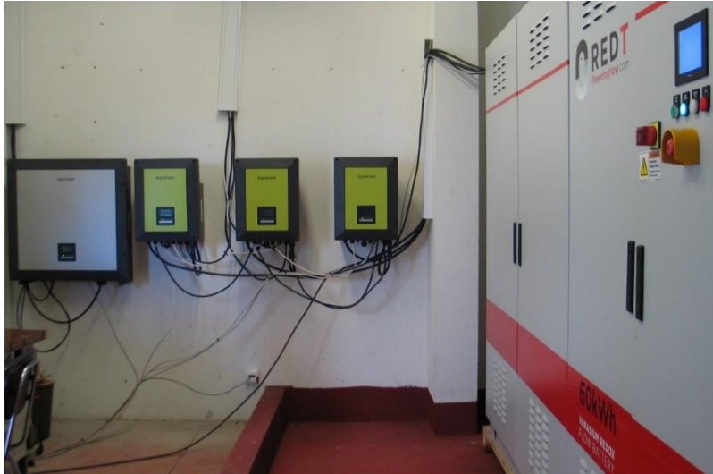
Figure 3. VRFB (right) and the inverters (left).
