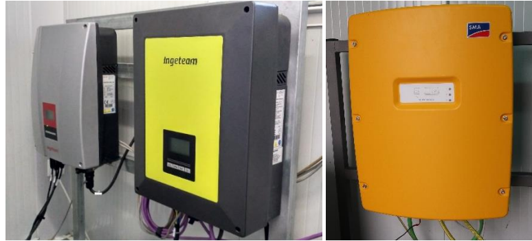
Figure 21: Inverters at the LIB microgrid: PV inverter (left), EMS Home bat. inverter (center) and SMA bat. inverter (right)
