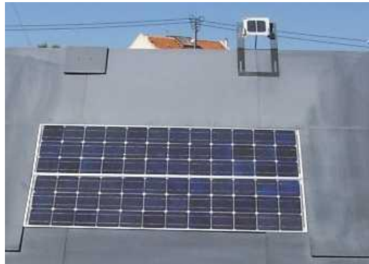
Fig. 7. PV system formed by two monocrystalline solar modules connected in series.
