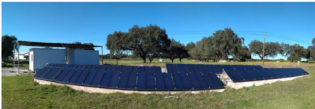
Figure 22: Ground installed PV strings connected to the Li-ion bat. microgrid
