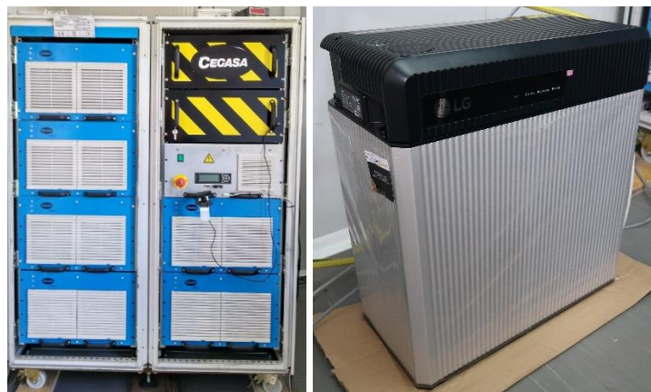
Figure 20. Li-ion batteries of the microgrid: Cegasa battery(left) and LG Resu10 battery (right)
