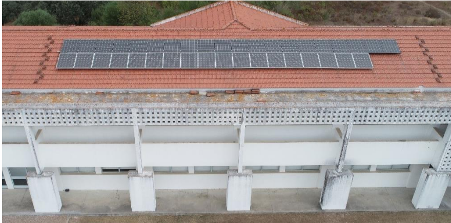
Figure 8: VRFB Microgrid rooftop PV system
