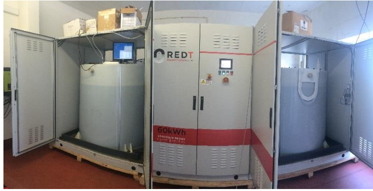
Figure 12. VRFB at UEvora. On the left and right the electrolyte tanks are visible, in the middle, the control panel and behind it the stack (not visible).
