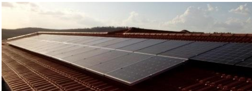
Figure 2. Roof mounted PV system.
