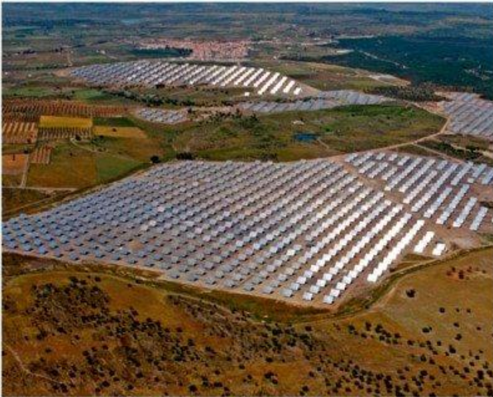
Photovoltaic Solar power plant in Moura, Portugal
