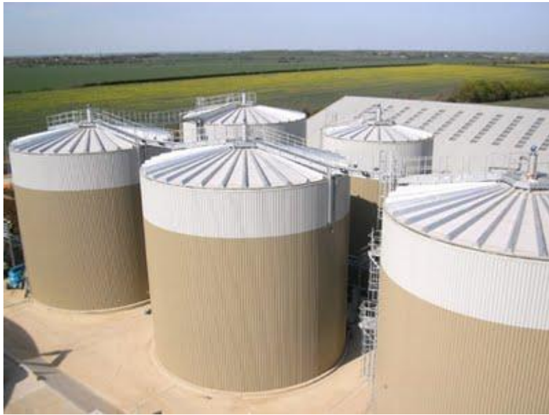
Image III Anaerobic Digester plant in Sweden
