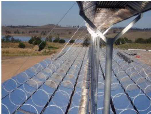
Fig. 3.1: One LFR system (AUSRA) with mirrors facing the absorber constituted by a series of tubes, placed next to each other.
