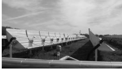
Fig. 1. Solar collectors (one of the twenty rows).
