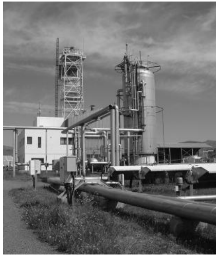
Fig. 2. Oil storage tank.
