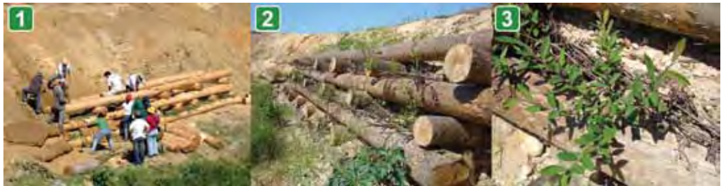
Figure 5.1.24 Construction of the cribwall to prevent erosion (1) general aspect (2) detail following budding (3) (Photos: Regina Carriço, 1 and André Fabião, 2 and 3).
