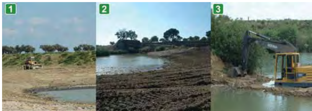
Figure 5.1.20 Final phase of work (1 e 2) and problems with submergence of heavy machinery due to the extreme underwater slopes (3) (Photo: Ana Mendes).
