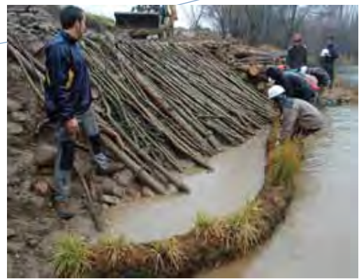
Figure 4.5.4.3 Brush mattress construction with willow poles and a vegetated fibre roll at the base. Ter river in Salt (Girona, Spain) (Photo: J. Bosch).
