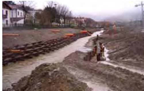
Figure 4.5.5.4 Construction of a log cribwall in an urban stretch. Artia stream in Irún (Guipúzcoa, Spain) (Photo: Paola Sangalli).
