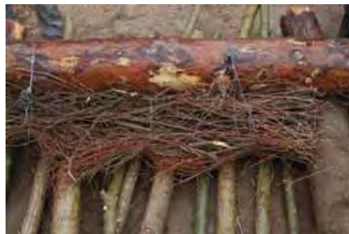
Figure 4.5.1.4 A fascine serving as a fine material retention structure in a log cribwall (Photo: J. Bosch).
