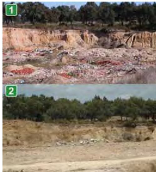
Figure 5.1.6 General aspect of the work area before (1) and after the clearing operations (2) (Photo: Ana Mendes).
