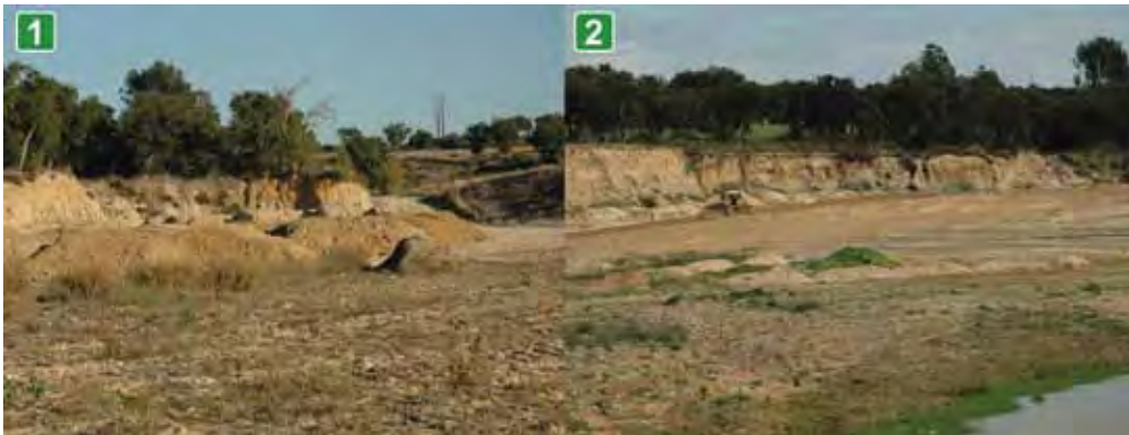
Figure 5.1.9 General aspect of the topsoil (1) and spreading over the site (2) (Photo: Ana Mendes).
