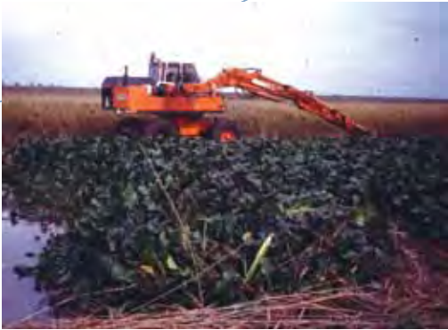
Figure 4.6.2 Hydraulic digger with a cleaning bucket in operation on a channel bank (Photo: I. Moreira).
