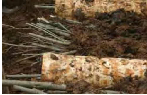
Figure 4.5.5.3 Willow cuttings placed in the crib wall cells and covered with soil (Photo: Antoni Bonafont).
