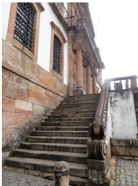
Figure 81 Pedra e cal masonry, used in the Museu da Inconfidência . We can as well see stones used in other elements, like the stairs, columns, lintels, sills, etc. Source: Gagliardi, 2019. 298
