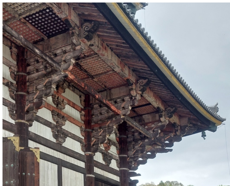
Figure 72 Great Buddha Hall ( Daibutsuden ), in Nara, Japan. It was the world's largest wooden building until 1998. The original structure dates from the 8th century, but it was destroyed twice. Today's temple was built in 1709 using the original techniques. Source: author.
