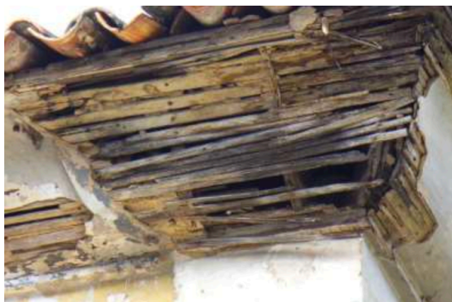
Figure 86 Use of the estoque in a cymatium in Ouro Preto. Source: Martins [2010] 304 .
