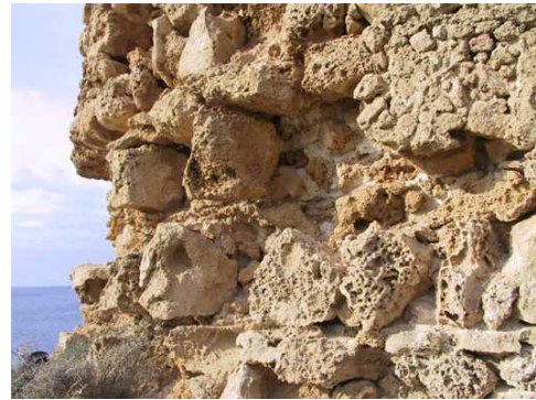
Fig. 4 - Inland side of the tower: evidences of tafones and flakings
