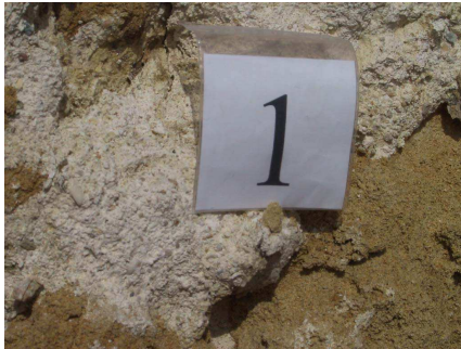
Fig. 6 - PSC-M1 sample – bedding mortar. The mortar is easy to breakage, whitish in color and full of shells inside.
