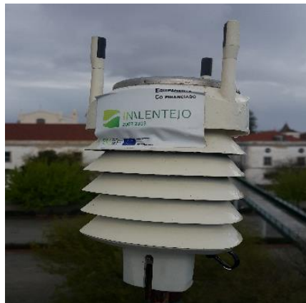
Figure 2.24 Vaisala weather station with temperature sensor.
