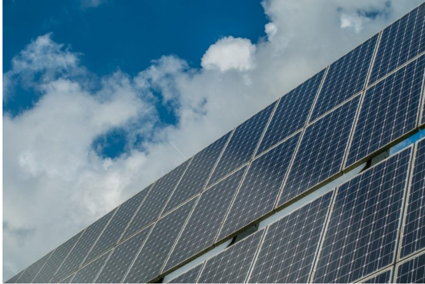
Figure 2.27 Cloud shadow on PV panels as time-dependent obstacle.
