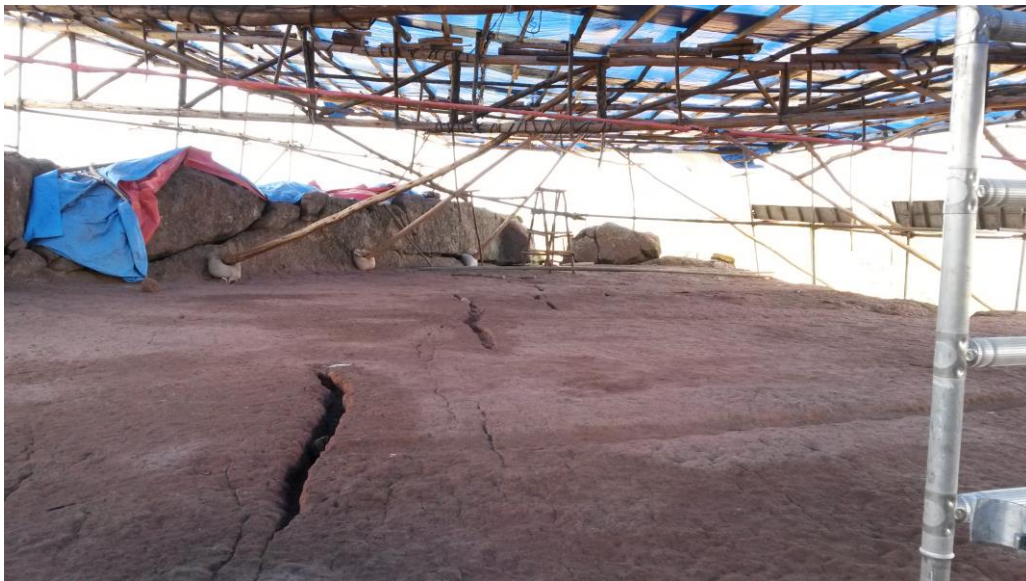
Fig. 2.3. The natural crack on Bete Gabriel's roof
